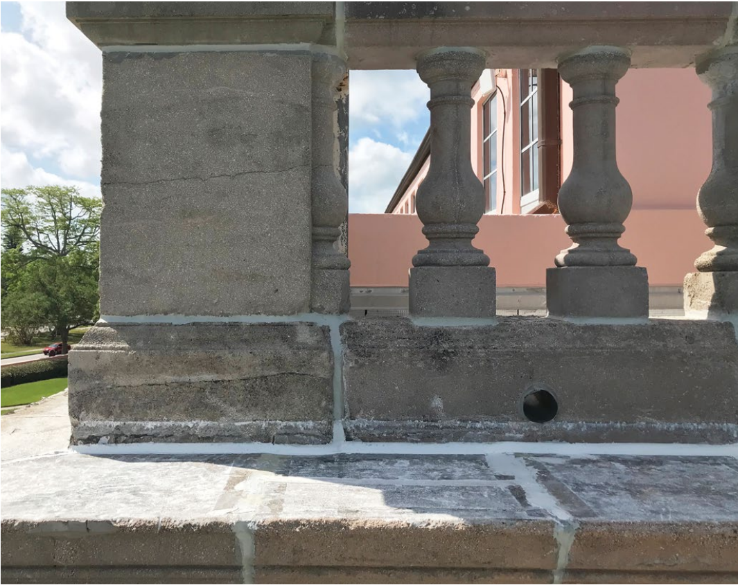
Figure 17. The balustrade consists of multiple prior campaigns of using cast stone to replace the natural stone. The effective match for the surface texture and color of the original stone allowed individual elements to be incrementally replaced only when they had failed, thus retaining the maximum amount of original material as long as possible. Photo: EverGreene Architectural Arts.
