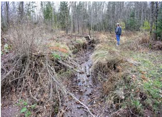
Steep road ditches and undersized culverts can activate headcutting and accelerate the loss of flood storage. Photo: WI Wetlands Association
