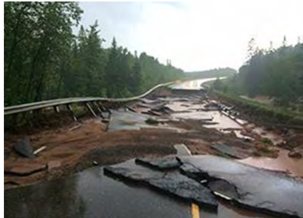
Road infrastructure damage in Ashland County
