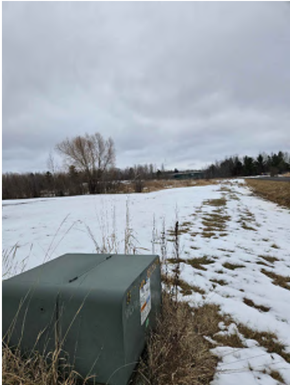
EXISTING POWER POLE / TRANSFORMER 3 SCALE: NTS
