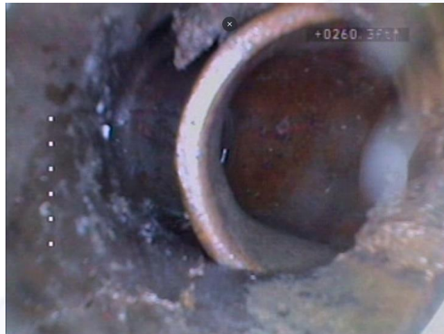
District 7: 304 13 th Avenue: broken connection between private sewer lateral and sewer pipe
