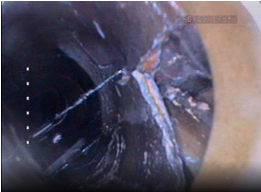
District 7: MH 472-471: hole in sewer pipe wall with infiltration
